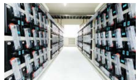
鉛蓄電池(1,152kWh)
